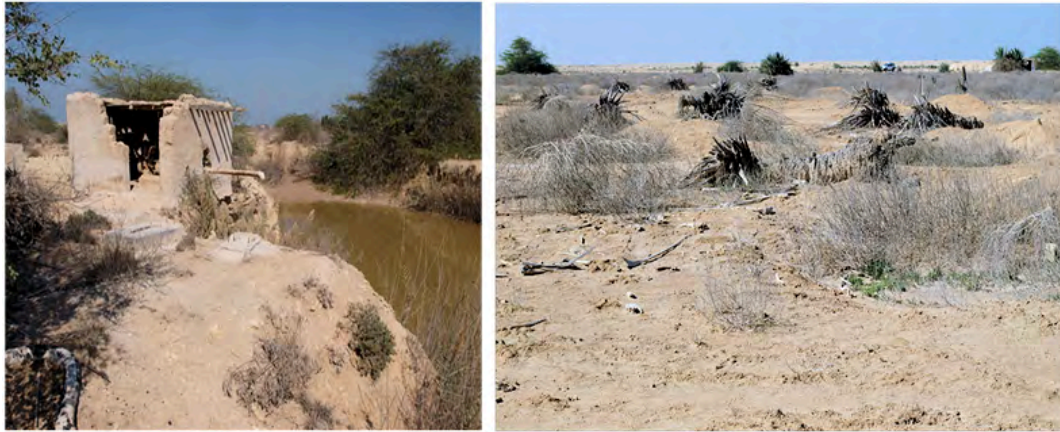
Figure 15. Abandoned pump house (left) near Al Thaqab on an irrigation pit showing the present a high water table. It was constructed for irrigation purposes, but rapidly become saline. Nearby dead date palms (right) attesting to the salinization of the groundwater in large nearby pumped pit-wells. (P.G. Macumber, 2014)
