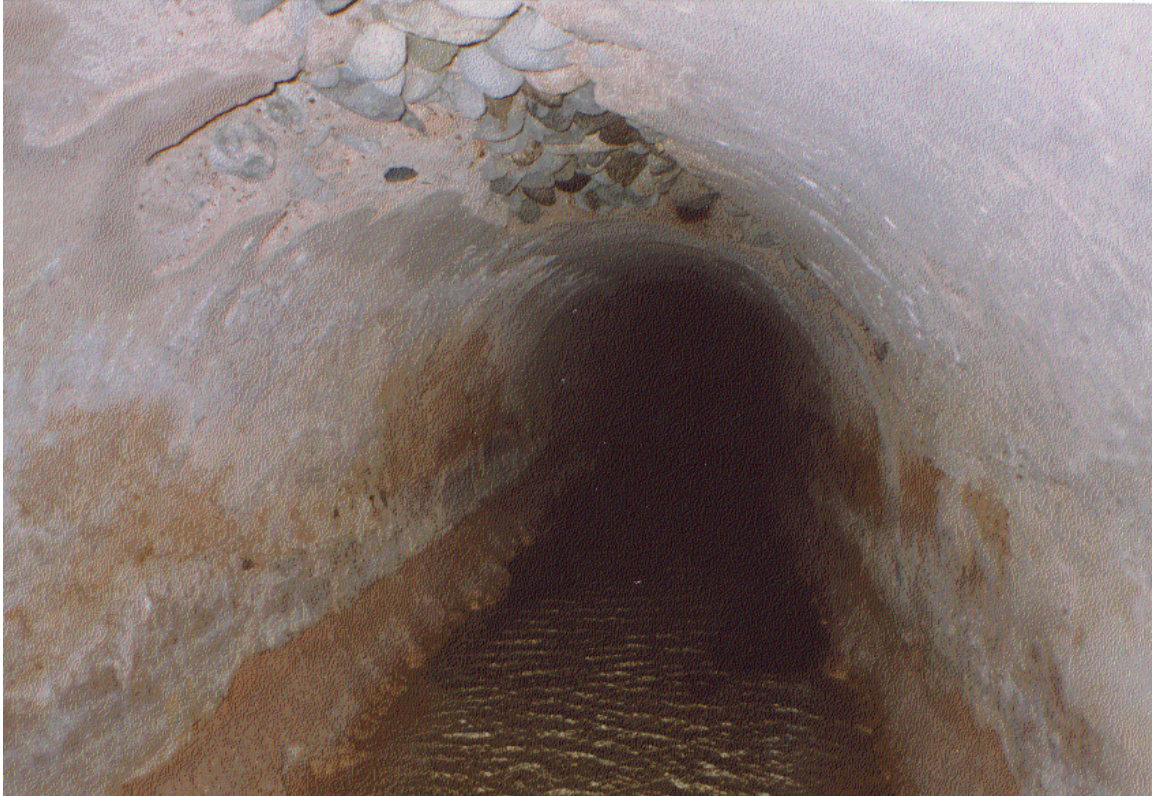
Figure 7. Interior of large daoudi falaj lined with clay and stones (nomination file, SP of Oman)
