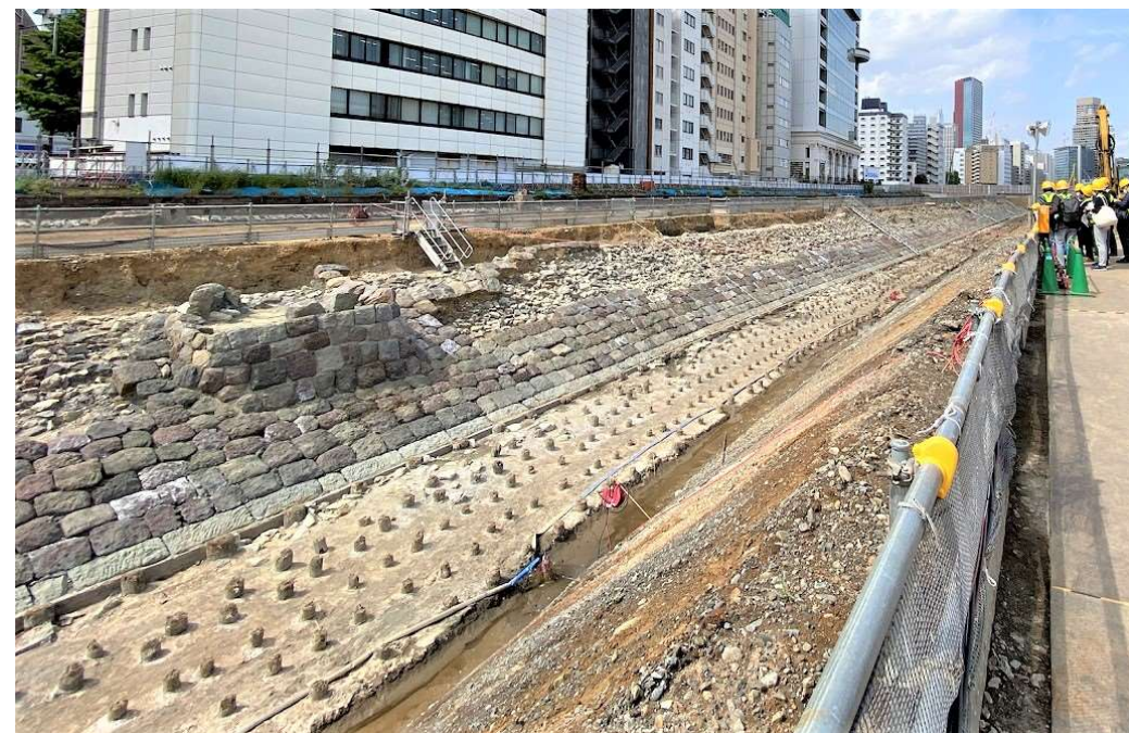
Extending embankment with the traffic-light base unearthed in Block 4 (from south), to be removed
